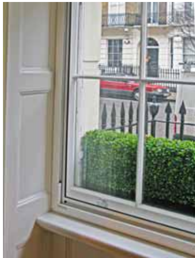
An example of a carefully incorporated secondary glazing system.
